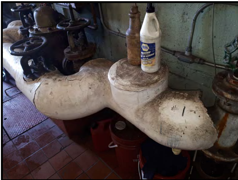
PHOTO # 6 Sample # ONR 1 : Asbestos-containing Elbow / Fitting Insulation on Cold Water Supply lines in Power House. (80% chrysotile asbestos)
