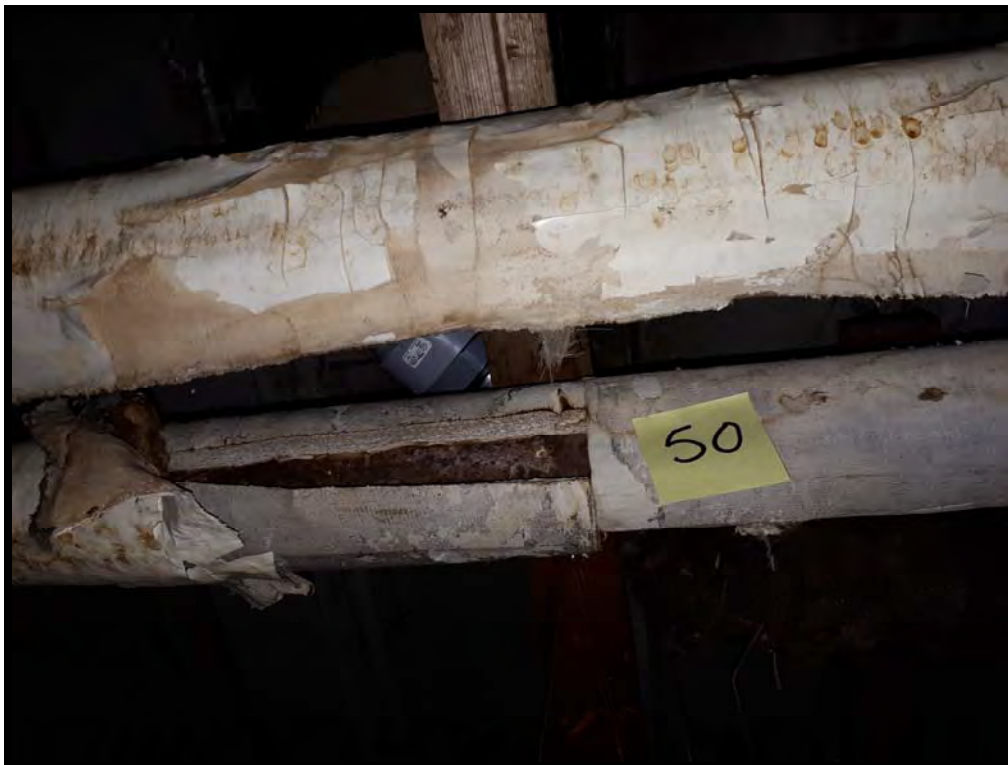
PHOTO # 32 Sample # ONR – 50 : Asbestos-containing Pipe Insulation (anti-sweat) on Heating lines in Diesel Shop - Room # 17. (70% chrysotile asbestos)
