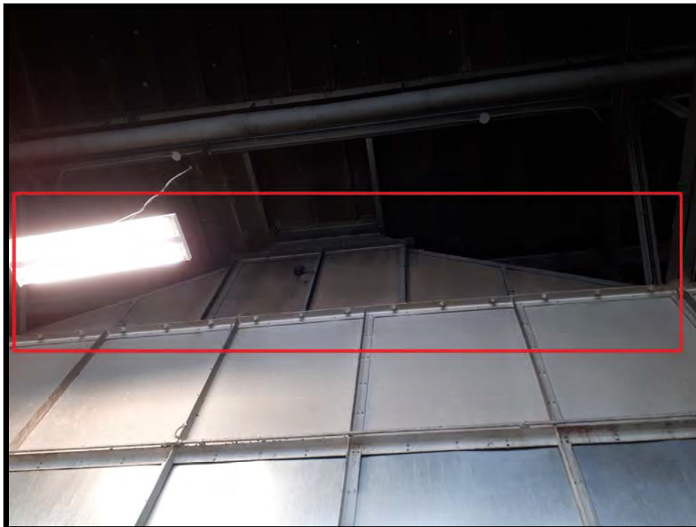
PHOTO # 43c Asbestos-containing “Transite” panels on upper part of exhaust hoods for locomotives in Diesel Shop – above Service Pits
