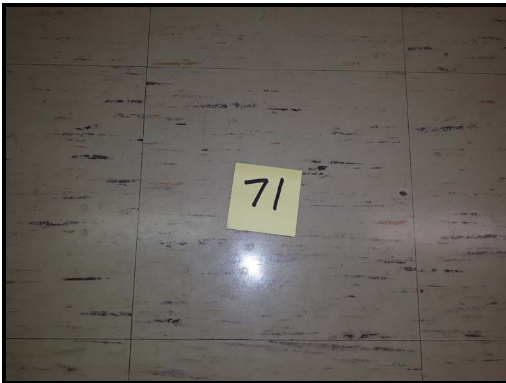
PHOTO # 42 Sample # ONR – 71 : Asbestos-containing 12" x 12" Vinyl Floor Tile in Car Shop - Room # G (25% chrysotile asbestos)
